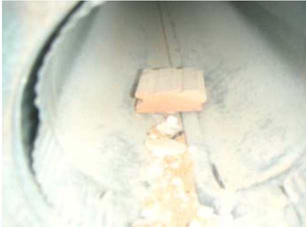
Construction debris in ducts.
