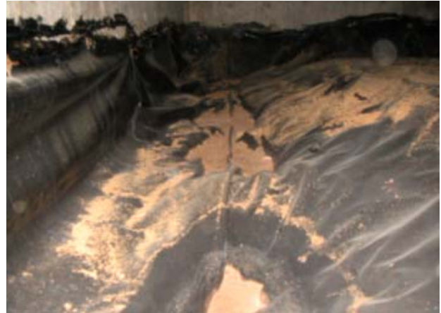
Sawdust and wood scraps on top plastic in crawl space.
