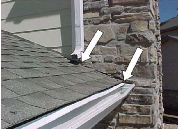
Missing kickout flashing.
