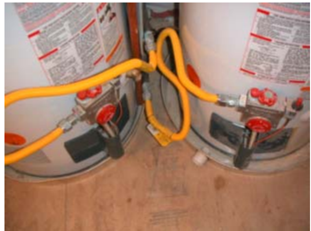
Discharge pipe missing at water heater drain pans.
