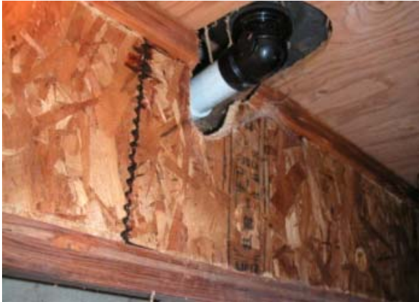
Joist flange cut under bathtub.
