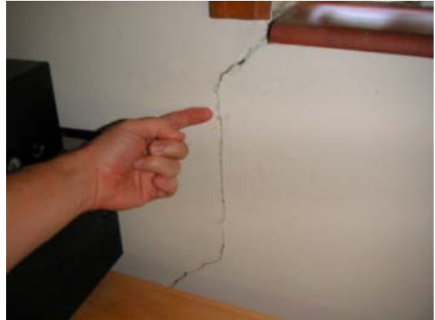
Wall cracks in rear addition.
