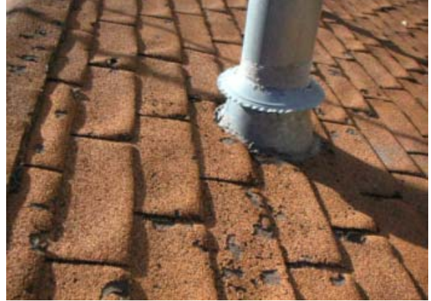
Worn out shingles.
