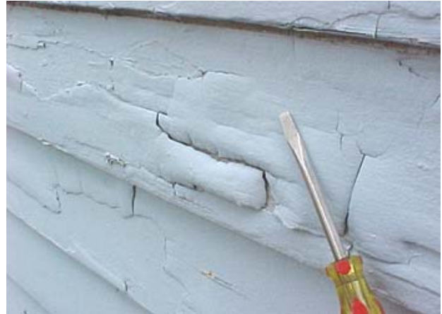
Peeling and cracked paint.
